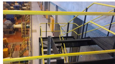
Painted Handrails and stairs in the engine room at Zuikerbosch (Rand Water).
