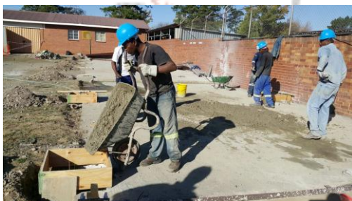
Preparation of the plinths for the building of a Warehouse at Rand Water Zuikerbosch
