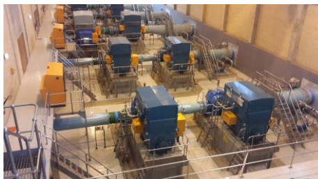
Painting of a water pumping engine room at Zuikerbosch (Rand Water).
