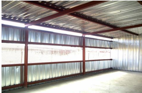
Manufacturing and erection of a steel structure for a government project in Coleen (Free State).
