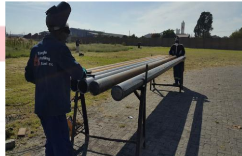
Preparation of 150mm OD x 8mm thk x 6m Long Steel Pipes for Bill Board Frames
