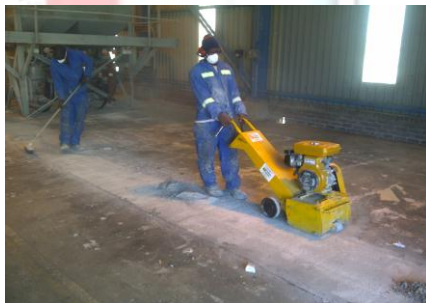
Preparation of the concrete floor for epoxy painting in a chemicals storage plant at Panfontein (Rand Water).
