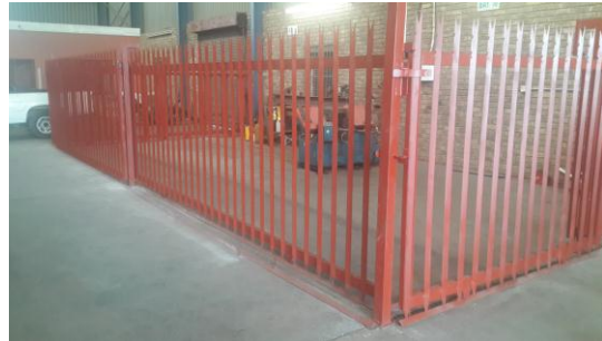
Manufacturing and erection of a double rail pallisade cage for ArcelorMittal Vanderbijlpark.
